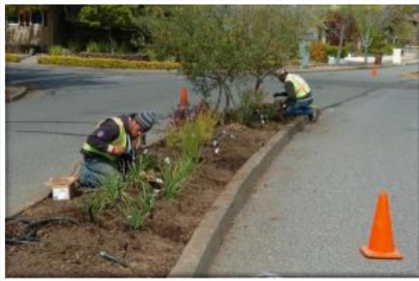
Eduardo Garcia (left) and Hector Tomayo put in irrigation pipes in the median of Peacock Dr. near Pt. San Pedro Rd. in the Peacock Gap neighborhood of San Rafael. This is a city-neighborhood partnership to reinvigorate the medians and addresses a long-standing need with a shared financial responsibility. (LJ photo/Frankie Frost)
